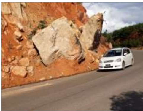
Figure 6 Rockfall site at the side of the road. (N 25° 21' 35.8" and E 97° 45' 30.1")
