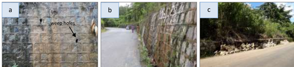
Figure 9 Retaining walls, which have been constructed by granitoids, along the Mtitkyina-Kanpetii car road; (a) weep holes (b) wall without weep holes (c) damaged wall.
