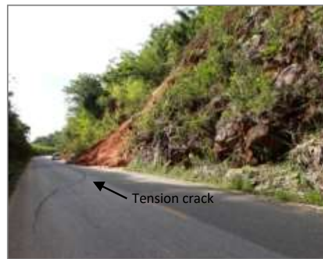
Figure 7 Forming tension cracks indicate to occur circular failure. (N 25° 21' 35.2" and E 97° 45' 27.1")
